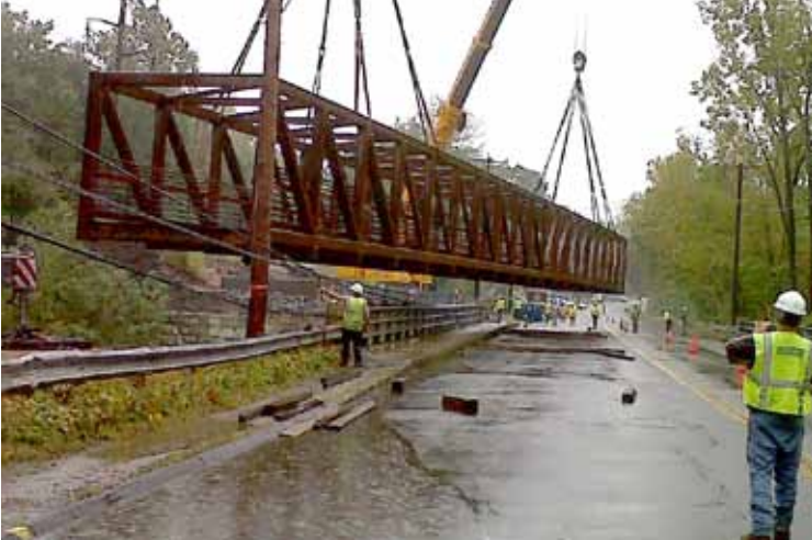
MassDOT workers repair a bridge over the Manhan River in Hampshire County as part of the Accelerated Bridge Program.
