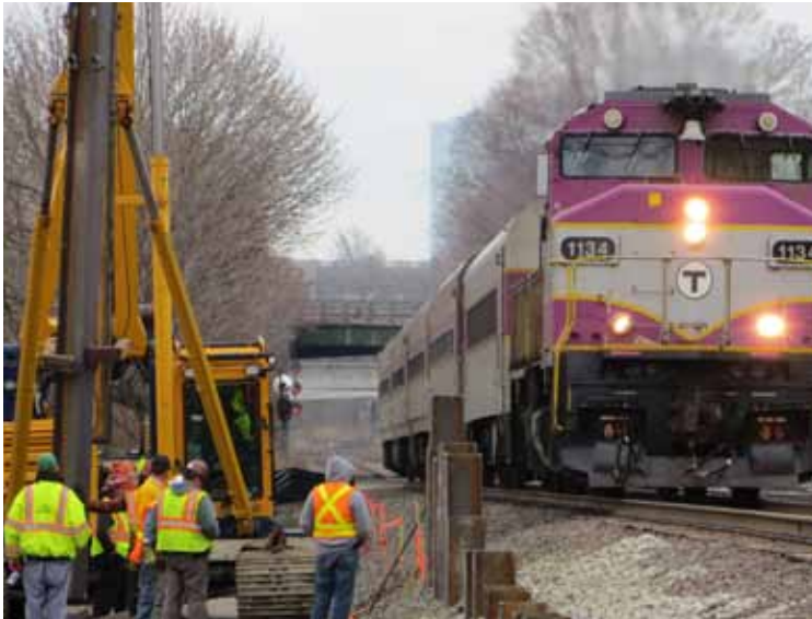
Work takes place on the MBTA Green Line extension in Somerville as a commuter rail train passes by.
